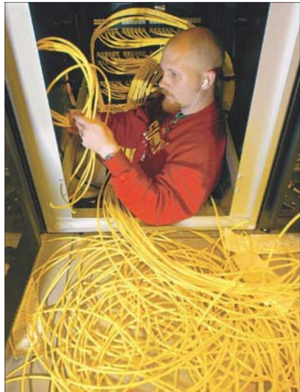
Kevin Essary installed wiring Aug. 29 at Progressive's data center under construction in northern Colorado Springs. The Economic Development Corp. hopes more data centers come to the city. (JERILEE BENNETT, THE GAZETTE)
